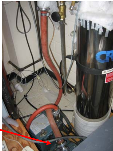
Mechanical pump for dewar (purging)
